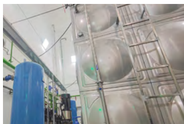
100 liter concentrated water treatment equipment for building 1 in the park
