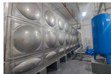
180-litre concentrated water treatment equipment for building 2 in the park (not yet put into use)
