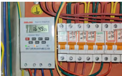
Timing switch of lighting system for underground parking lot of Building 1 in the park
