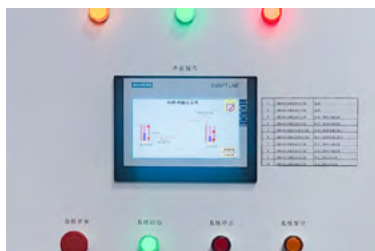
Concentrated water treatment system of building 1 in the park
