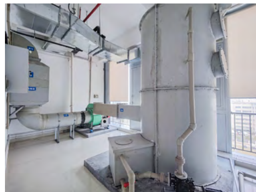
Activated carbon waste gas treatment system
